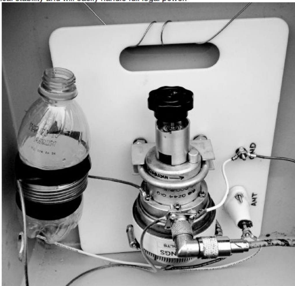
Figure 3 — Mounted on a common plastic kitchen cutting board, the heavy-duty vacuum variable capacitor is connected in series with the load. An improvised 3\ \mu\text{H} inductor is attached to convenient points on the capacitor and to the circuit's common ground point.
