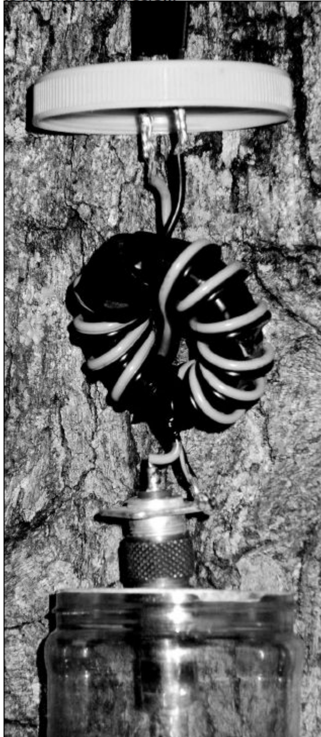
Figure 4 — A version of the balun with the crossover winding. Notice how the input and output connections are in line with the feed lines.
