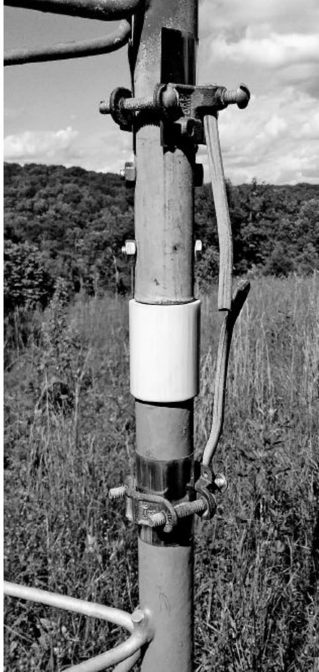
Figure 1 — A 300-series stainless-steel shim between a bronze ground clamp and galvanized tower leg protects the zinc layer and the clamp.
